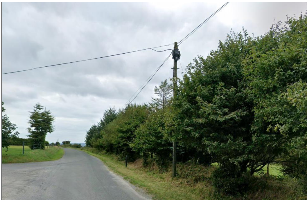
Figure 17. Fibre on Pole at Entrance to Carrondavderg Telecoms Mast Site
