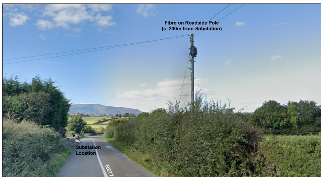
Figure 21. Fibre on roadside pole c. 200m from Cooltubbrid Substation
